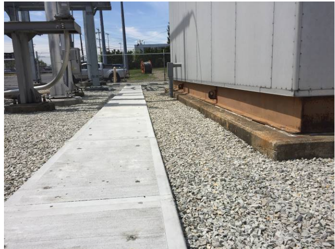
Figure 2 – UG Cable Pump House Located in Floodplain
