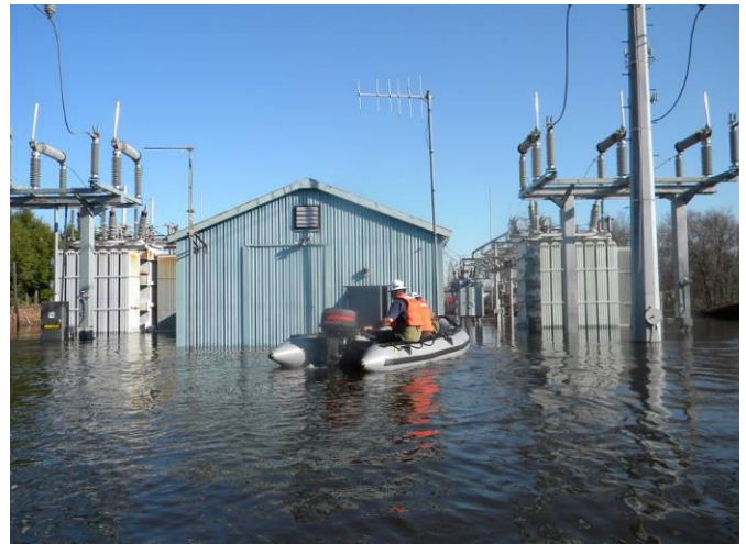
Figure 1 - 2010 Flooding of RI Substation
